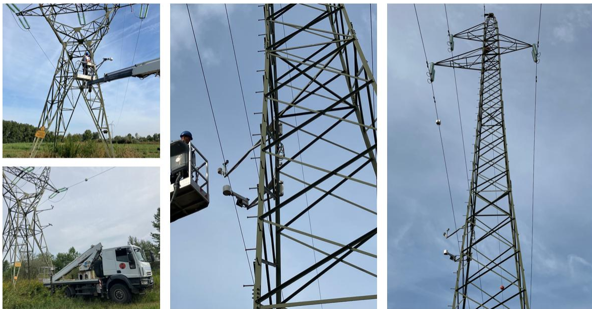
Figure 10 Hardware installation on the E.ON grid
