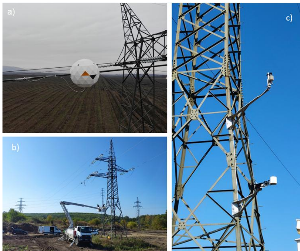
Figure 2 - Installation of dynamic line rating equipment in the Hungarian distribution and transmission system: a) line monitoring sensor, b) weather station c) weather station [7]
